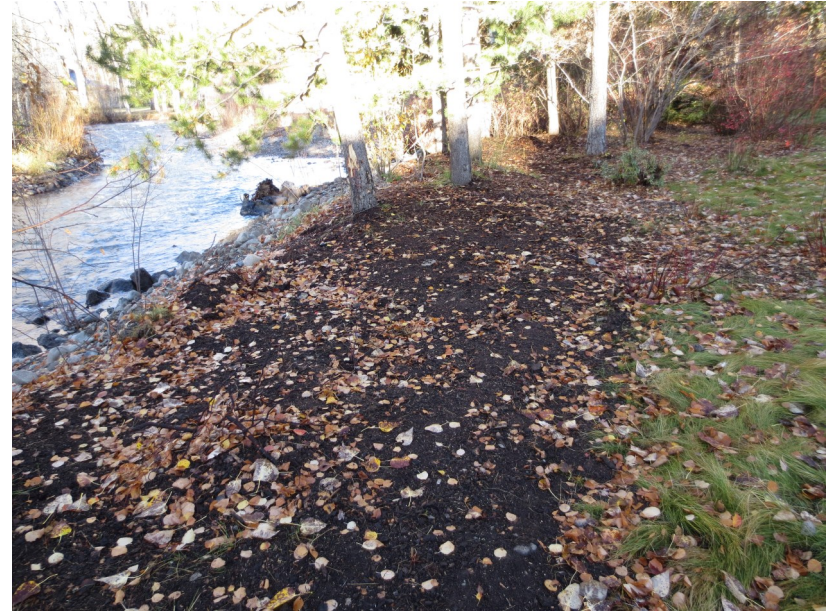
Two Most Northern Barbs and Toe Protection/Reseeded Area
