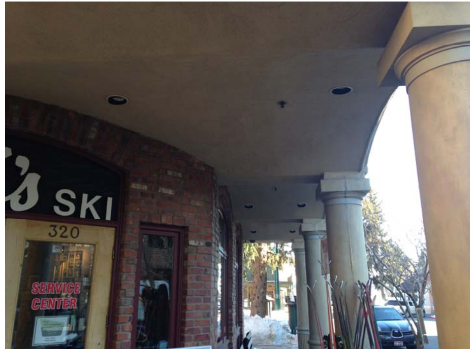
EXTERIOR LIGHTS @ FRONT COLONNADE
