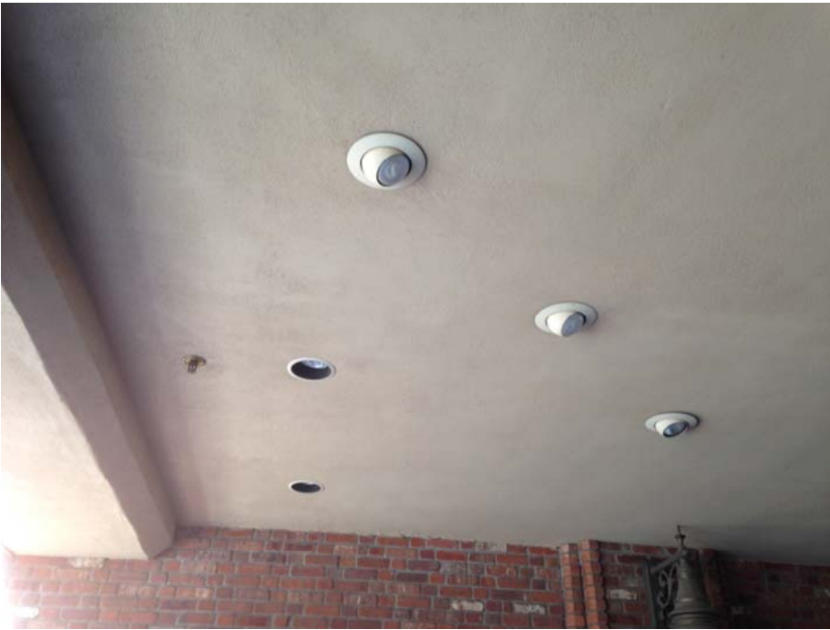
EXTERIOR LIGHTS @ PROPOSED ADDITION
