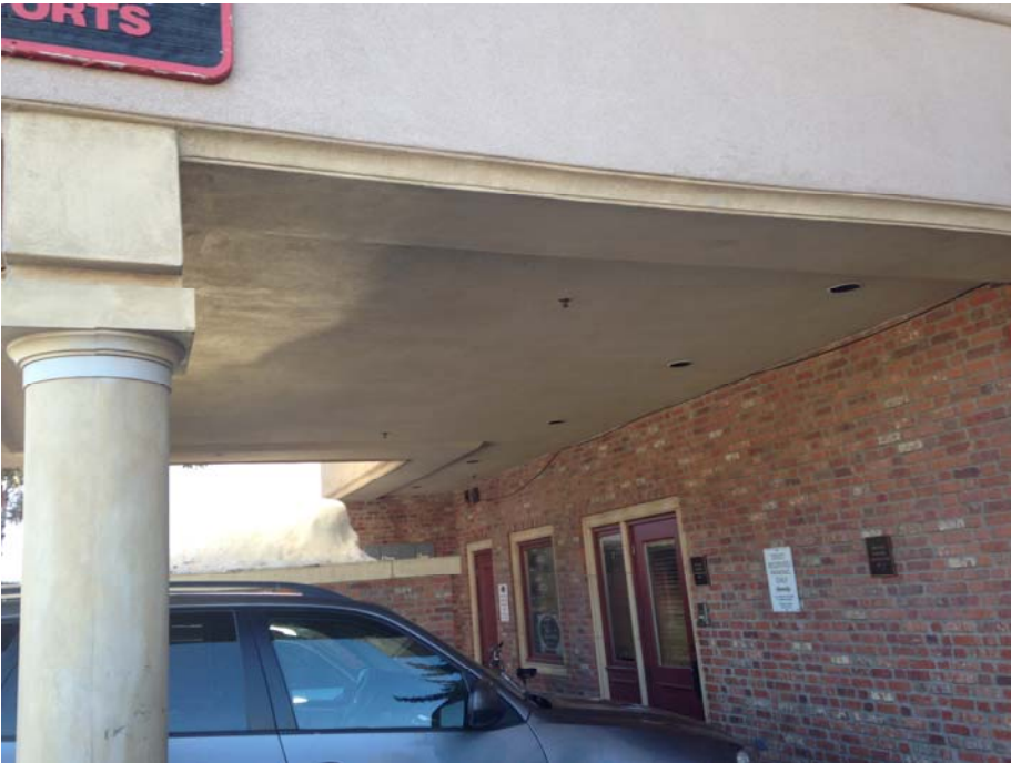
EXTERIOR LIGHTS @ CARPORT
